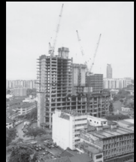
Abandoned construction site of residential towers in Kuala Lumpur (Pic.6)
